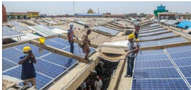
Solar panels on stalls of Sabon Gari Market
